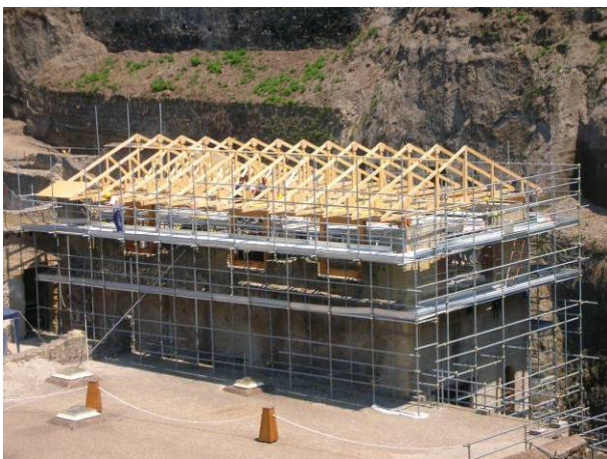
80% of dangerous existing roofing has been repaired and new shelters have been created
